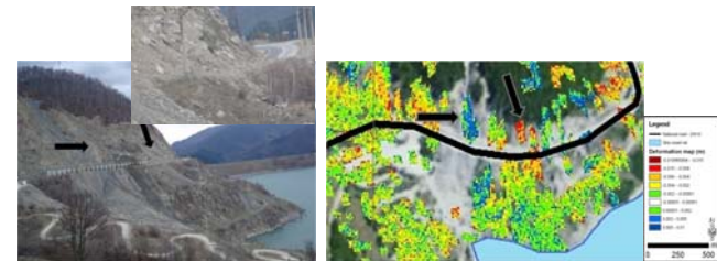
East bank landslide affecting a national road (left - photographs, right - deformation map)
